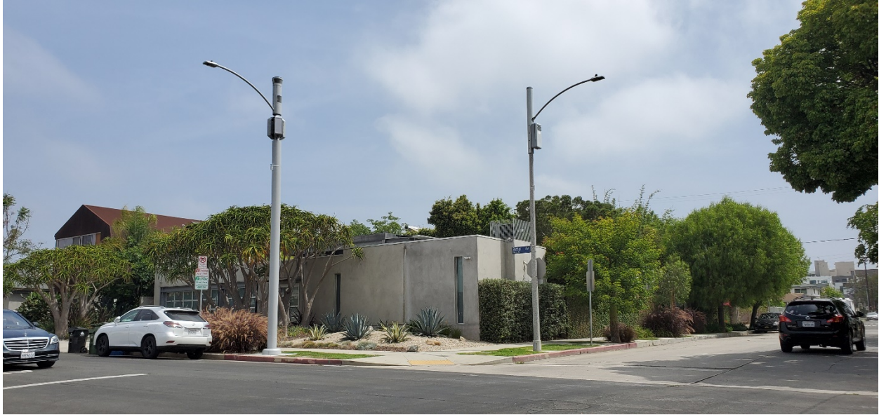
Figure 10: Single-carrier, two-band 5G site (left) on a light standard adjacent to a single-band 4G site (right) both in the right of way (Los Angeles, CA). Photograph by Dr. Jonathan Kramer.
