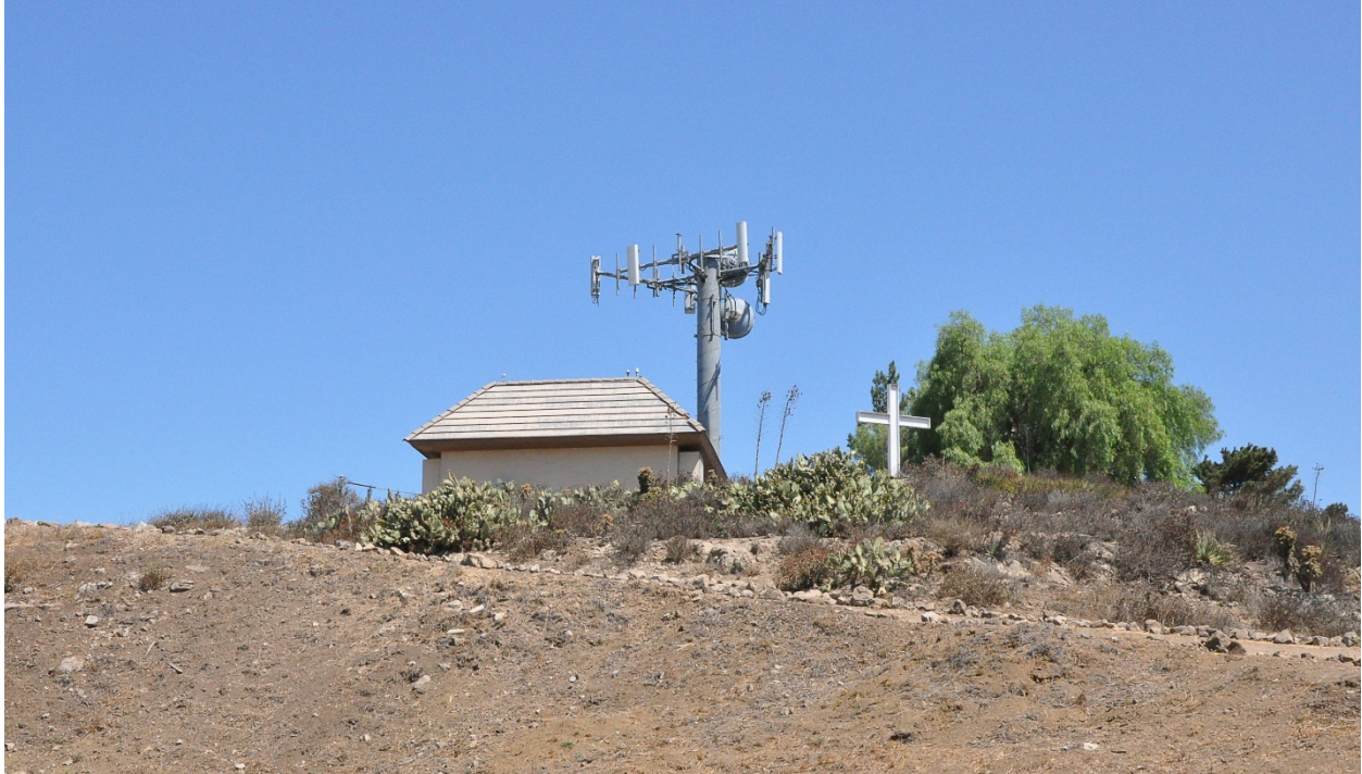
Figure 5: Multi-carrier 4G site (Thousand Oaks, CA). One carrier on the stub tower, and one with antennas inside the roof of the building. Photograph by Dr. Jonathan Kramer.
