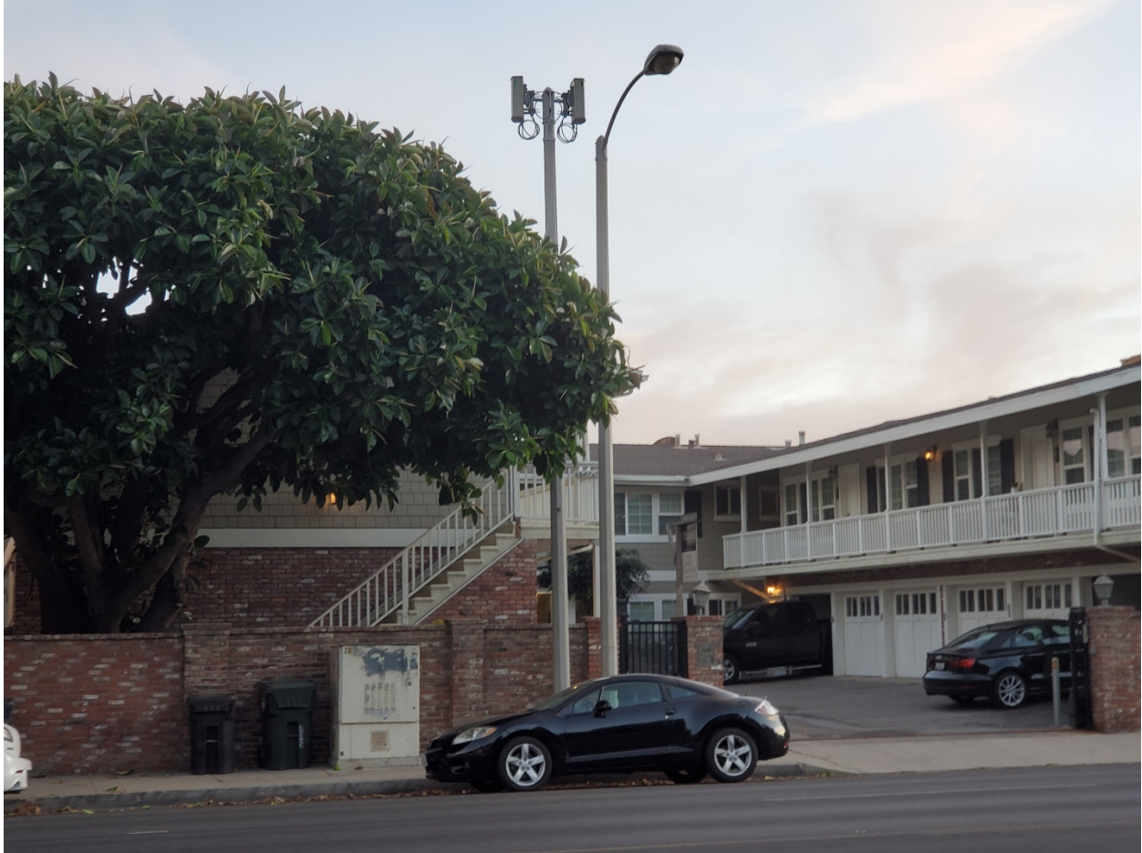
Figure 7: Single-carrier 4G site on a freestanding pole in the right of way (Malibu, CA). Photograph by Dr. Jonathan Kramer.
