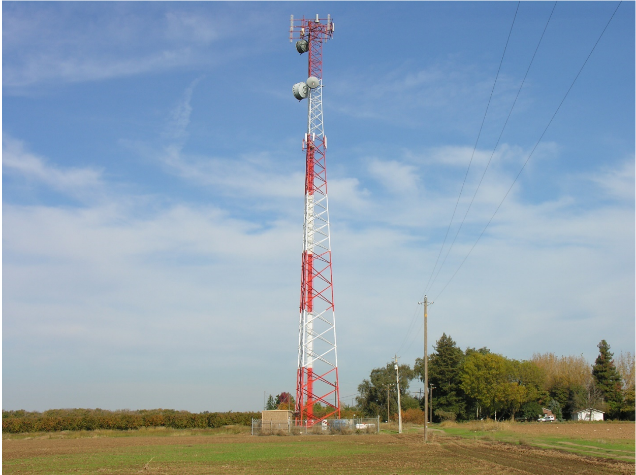
Figure 2: Self-supporting lattice tower supporting T-Mobile antennas (Gridley, CA). Photograph by Dr. Jonathan Kramer.
