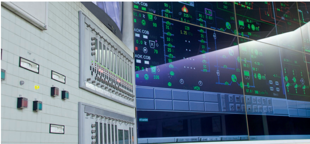
A modern power station control room.
