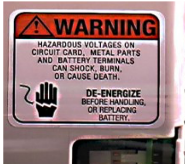
Label on side of smart meter
