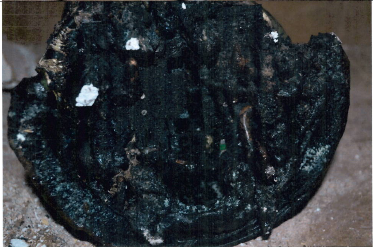
Above & below Smart meter
